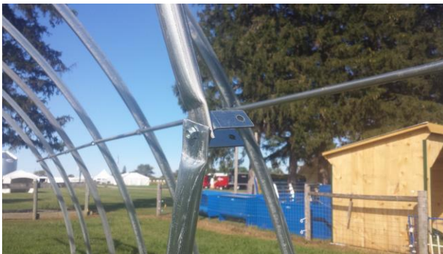
#23: The bottom end of one wind brace is tied to the top end of the next wind brace using the purlin clip already there
