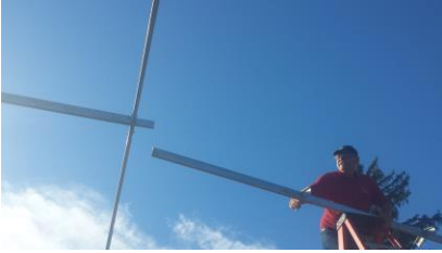
#14: connect the next section of ridge to the ridge starter at the end of the previous ridge section
