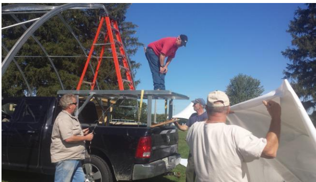
#42: all hands on deck, prepare to lift the cover onto the structure
