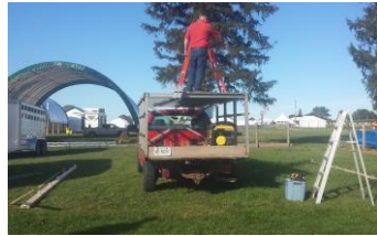
#2: measure and lay out the base (base bracket installation shown) and prepare scaffolding
